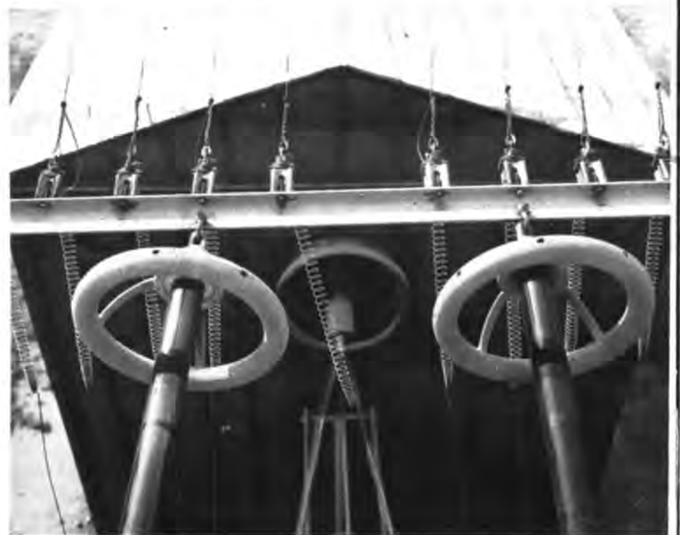
The first tuning house from the station, showing insulators with corona rings, feeders to the aerial and connection, through a large copper sleeve, into the tuning house. The rings are about two feet in diameter and the insulators about five feet long.
